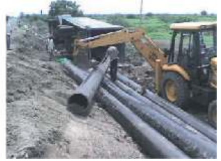
Damage to pipes due to accident
