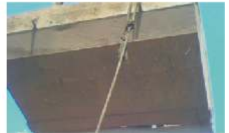
Grab Damage Survey
